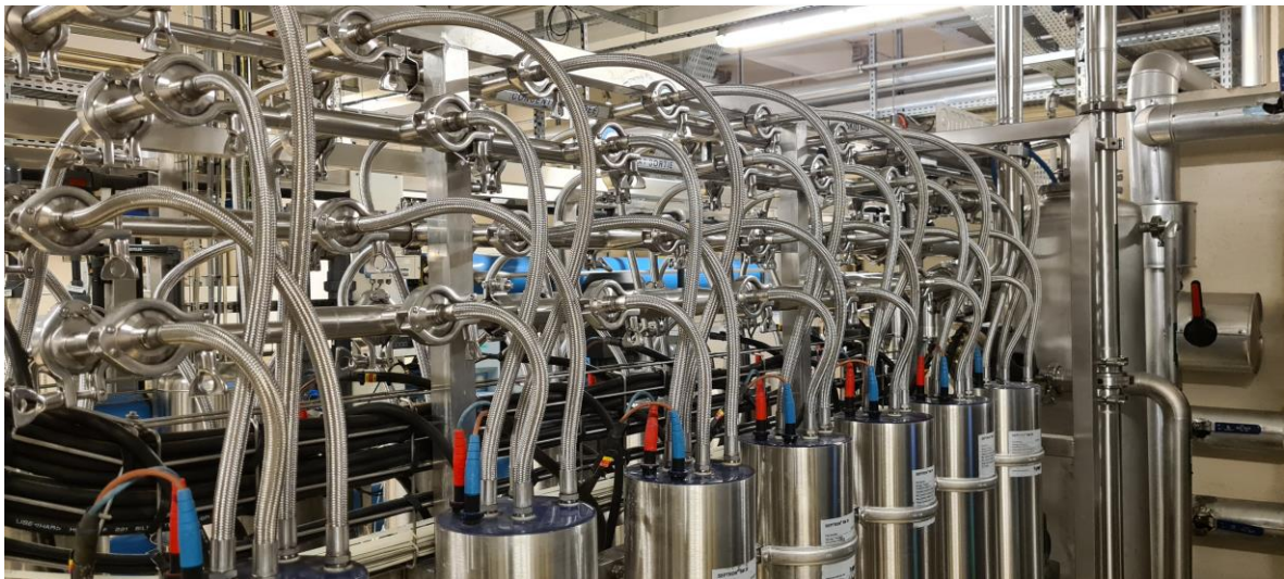
Water purification systems in our Production site of Val de Reuil, France
